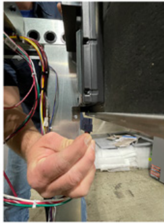
Disconnect the Molex plug in the bottom of the HMI.
